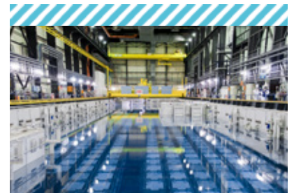
The spent fuel pools at La Hague can be used to store fuels pending reprocessing, in order to reutilise the radioactive materials they contain.
