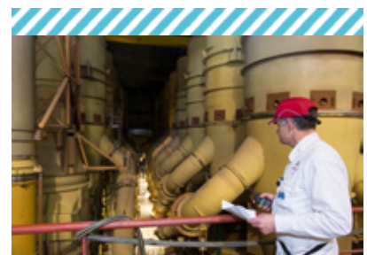
Intensive rinsing operations followed by air venting - decommissioning of the George Besse 1 plant
